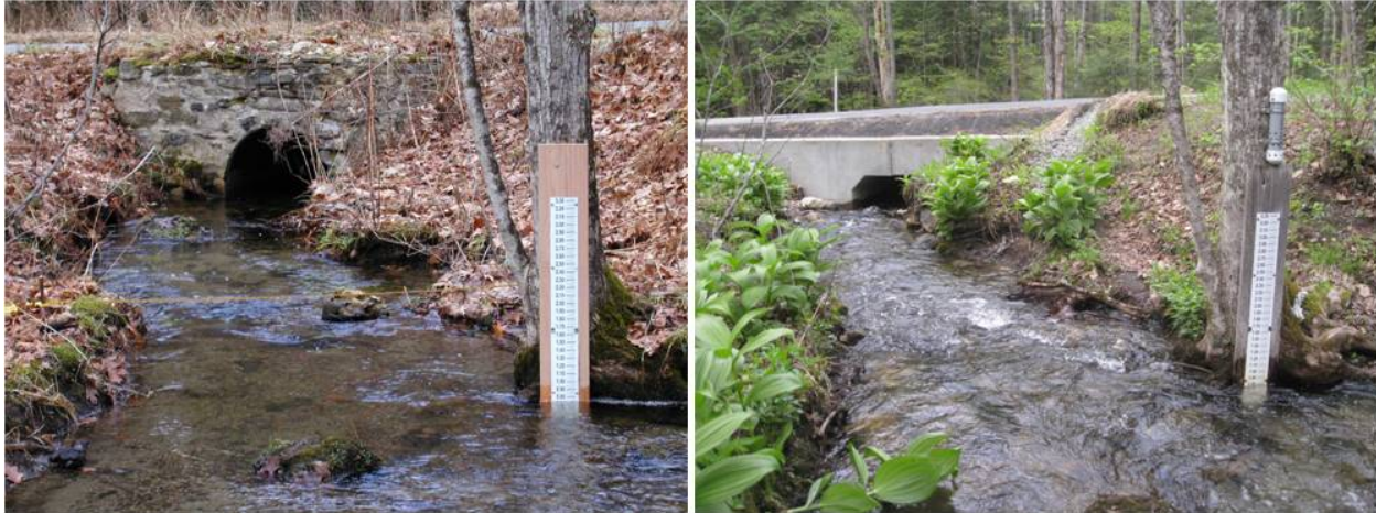
Figure 33. A culvert replacement downstream of a stream gage on Gulf Brook in Pepperell, MA caused enough of a channel change to necessitate a new rating curve.
