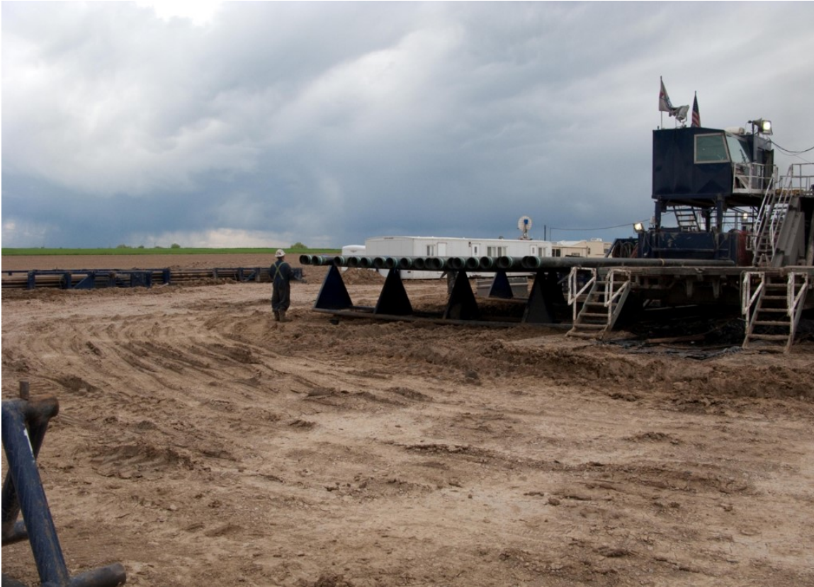
Figure 2-7. Sections of surface casing lined up and being prepared for installation at a well site in Colorado.
