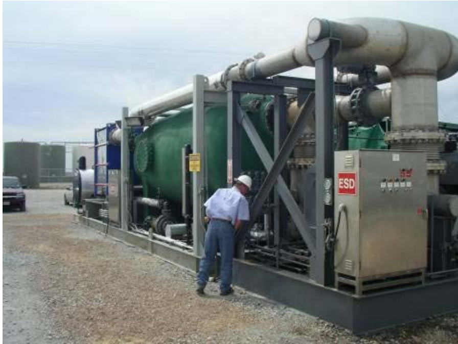
Figure F-4. Picture of a mechanical vapor recompression unit near Decatur, Texas.
