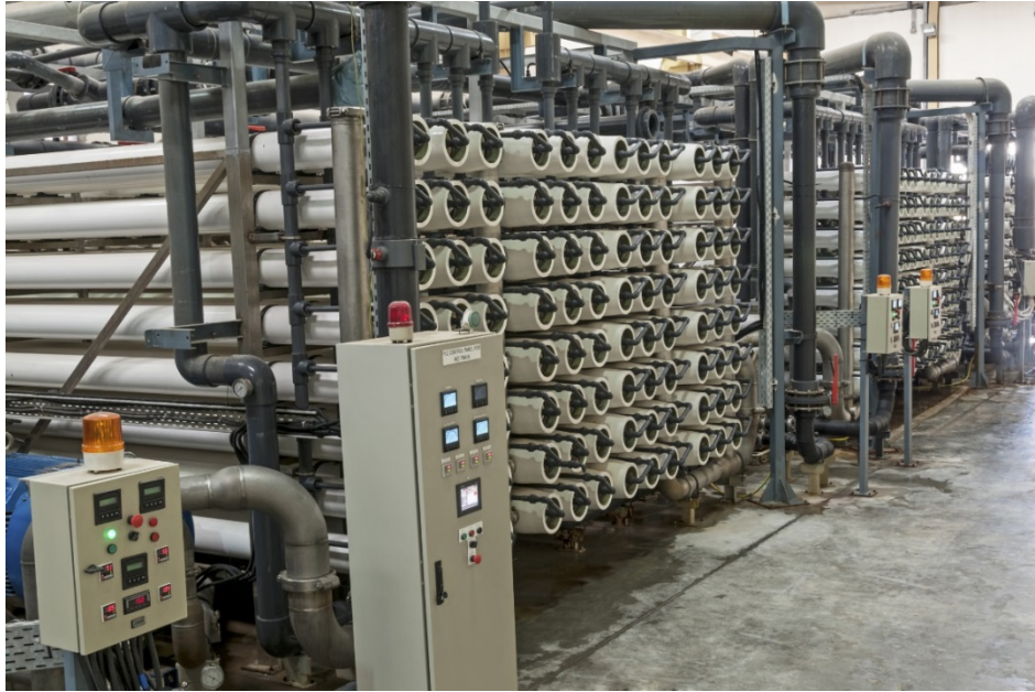
Figure F-2. Photograph of reverse osmosis system.
